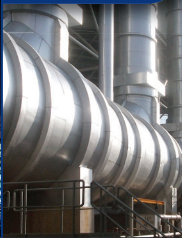
CCGT Power Station, Uskmouth Bespoke Acoustic Lagging System
